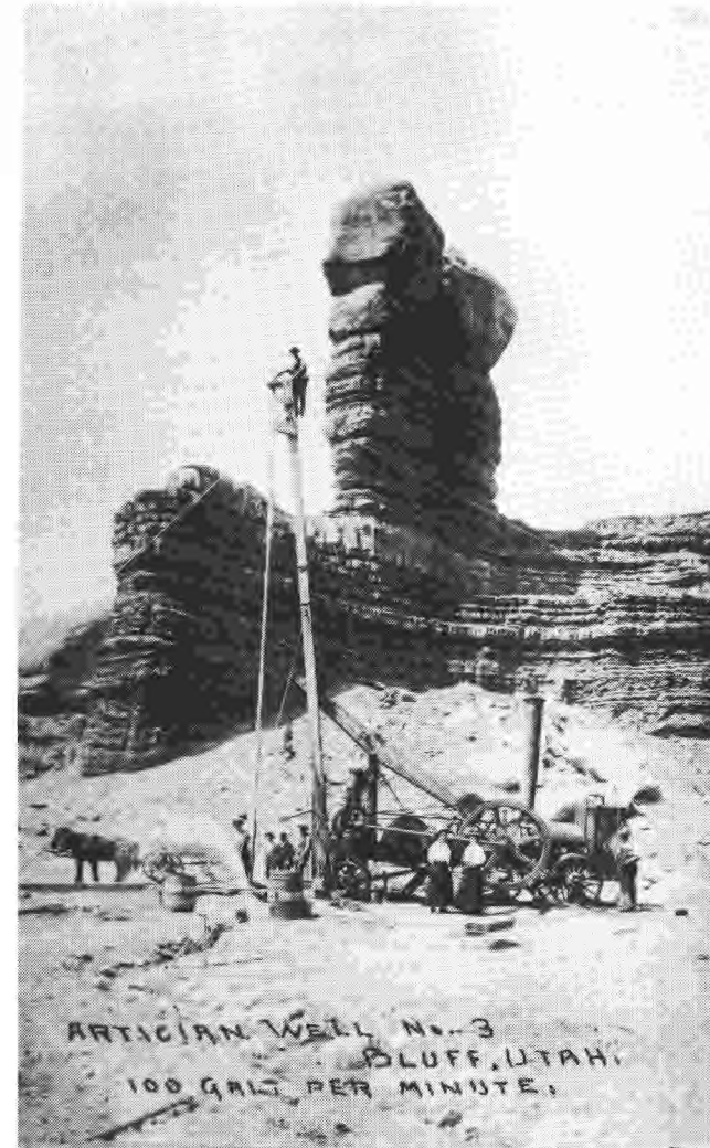
Artesian Well--North of Bluff City Pumps water at the rate of 100 gallons per minute.
